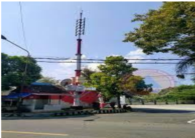
Figure 8. Damaged Tsunami EWS in Cuwik, Ploso Sub-district Source: Pacitan Regency BPBD (2025)
