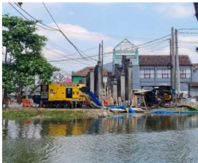
Figure 9. Pumping Flood Water Source: Researcher Documentation, 2025
